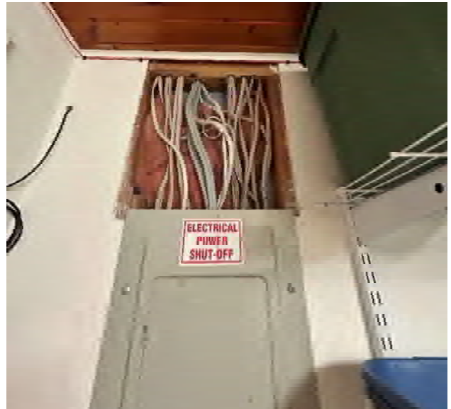
FIGURE 4.4.4: Existing panelboard and Romex wiring
