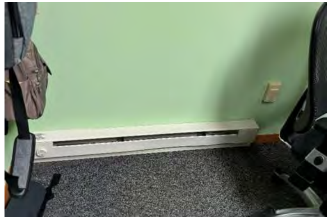
FIGURE 4.4.1: Baseboard heat at office
