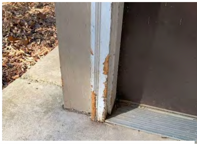
FIGURE 4.3.7: Wood trim damage at Workroom entry
