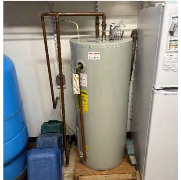
FIGURE 4.4.8: Existing water heater
