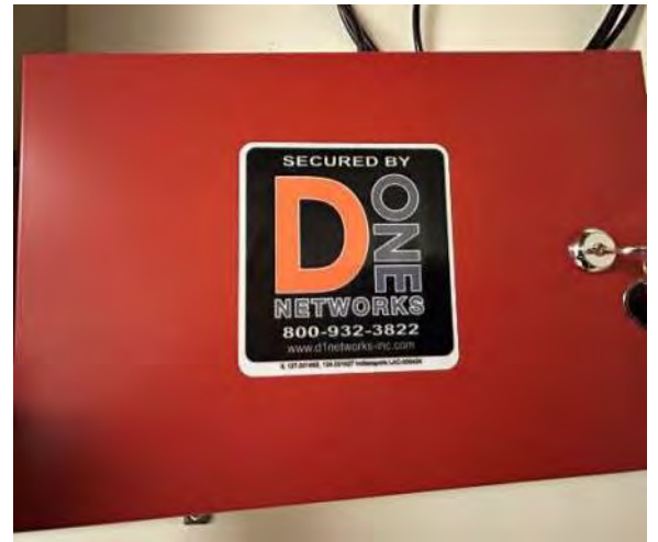
FIGURE 4.4.7: Security panel in janitor/mechanical room
