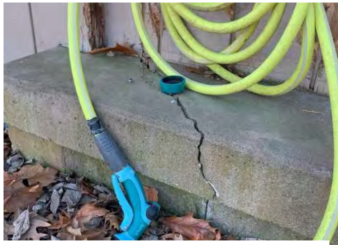
FIGURE 4.3.6: Cracking at slab/foundation wall, NW corner
