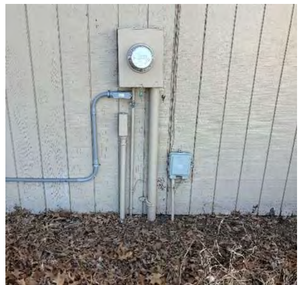
FIGURE 4.4.5: Electric meter mounted on building's east side
