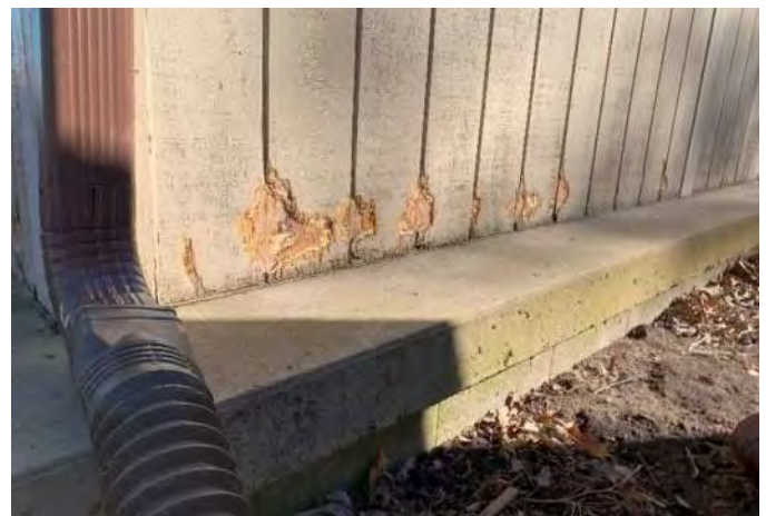
FIGURE 4.3.3: Wood siding deterioration at west side
