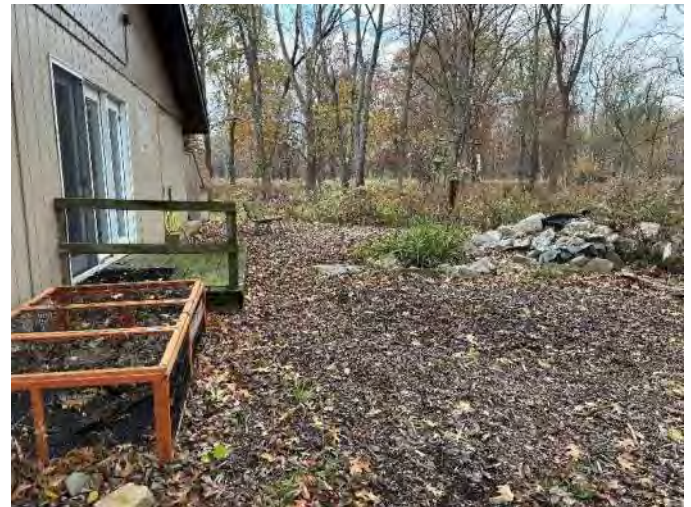
FIGURE 4.1.2: North side of the nature center. Water feature is non-functioning
