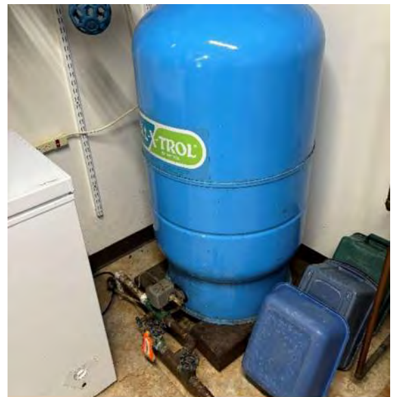
FIGURE 4.4.9: Pressure tank for well water
