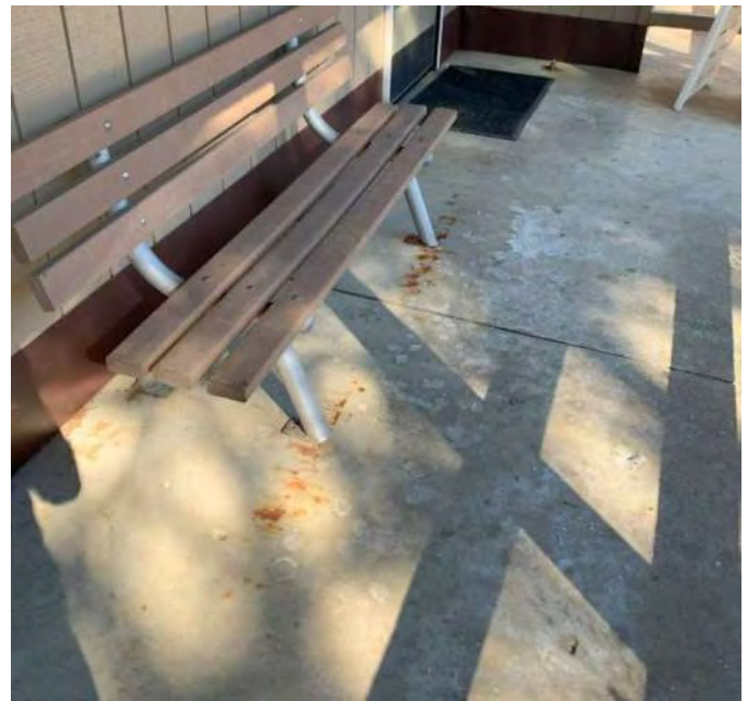
FIGURE 4.3.2: Existing condition of concrete at south entry
