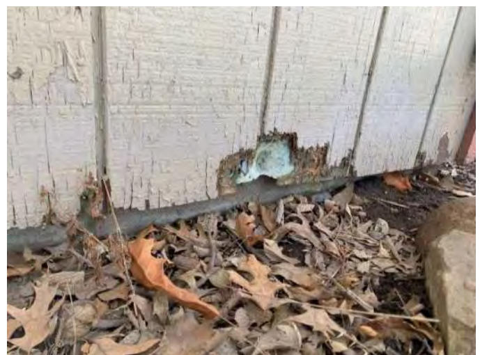
FIGURE 4.3.4: Wood siding deterioration at east side
