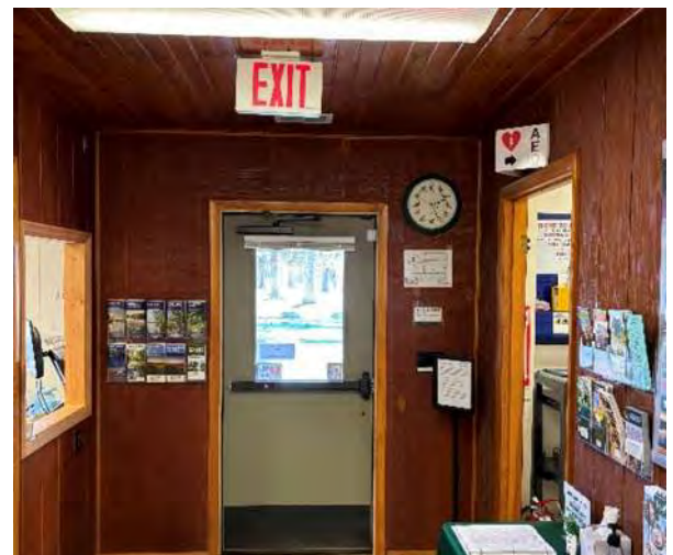
FIGURE 4.4.6: Emergency exit sign and typical surface mounted light
